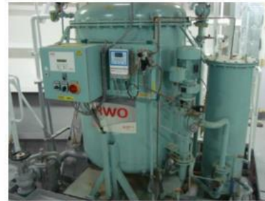
Oily Water Separators (OWS)
