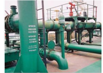
Venting Systems on Oil Tankers
